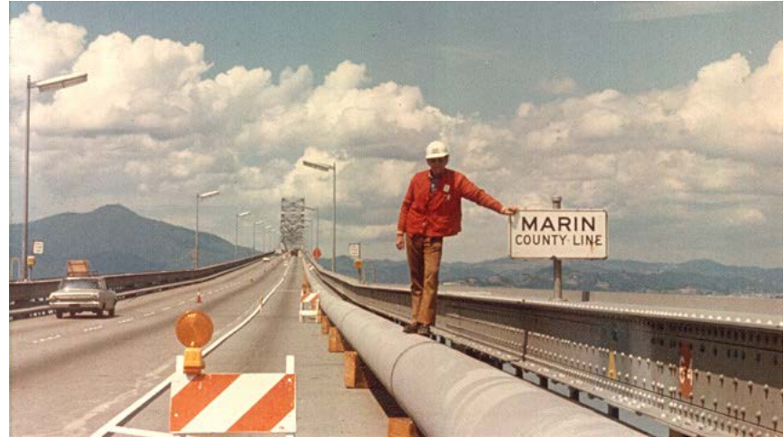
During 1976-77 drought, Marin County had to build a pipeline across the San Rafael-Richmond Bridge
