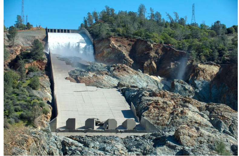
Oroville Spillway damage in 2017. Photo: DWR
