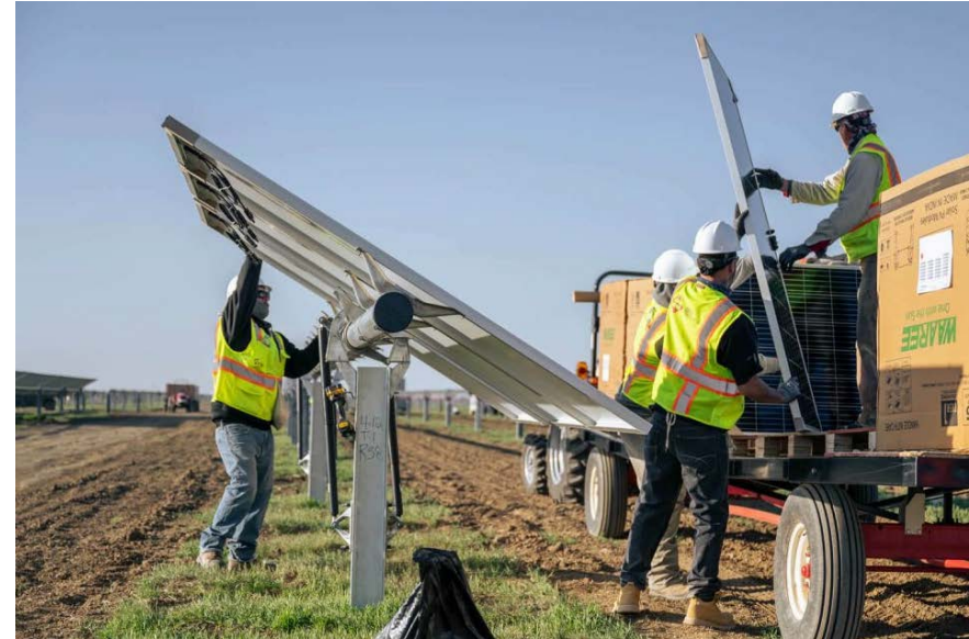
Aquamarine Westside Solar, SOLV Energy
